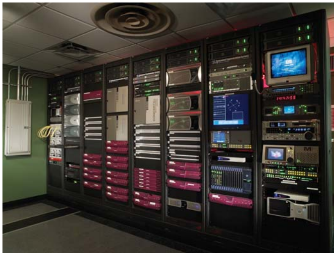
University of Miami equipment room with state-of-the-art broadcast products, including Avocent AMX5121 user stations and AMX5000 KVM switch.
